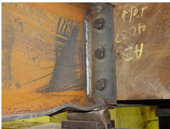
Close-up flange buckling (north girder)
