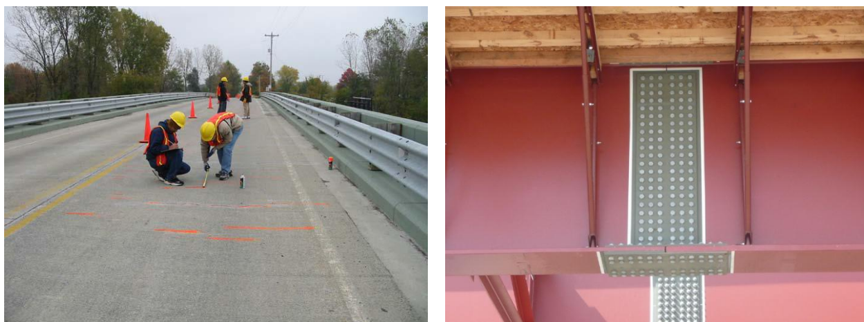
Figure 1-1. Example of mapping cracks in the concrete deck and steel girder splice.
