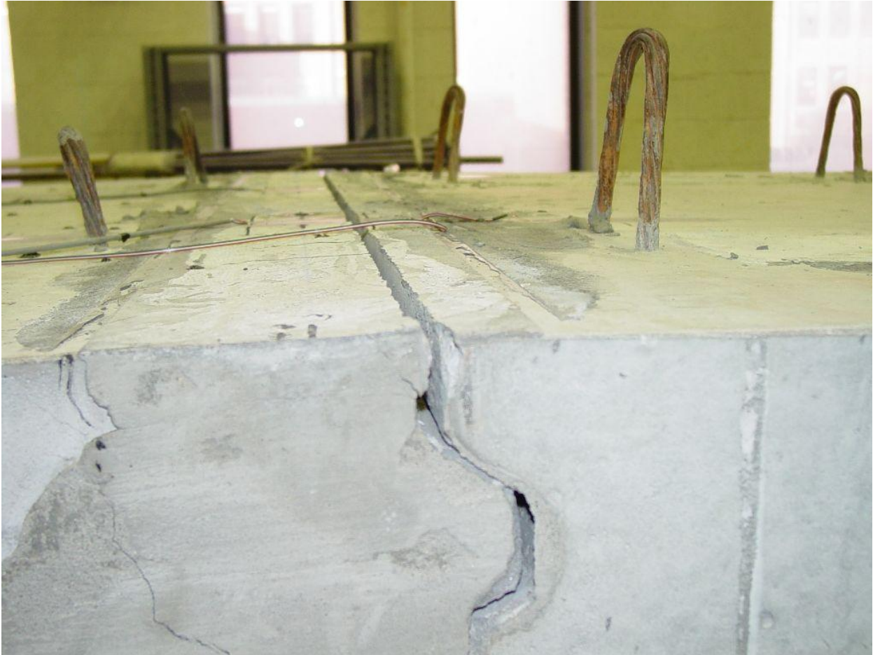
Figure 4-31. Crack at the closure region due to tensile force over interior support
