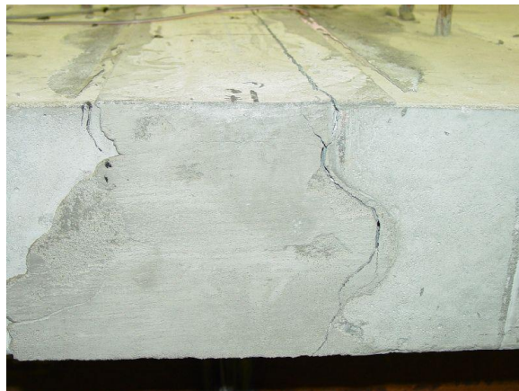
Cracking at closure region
