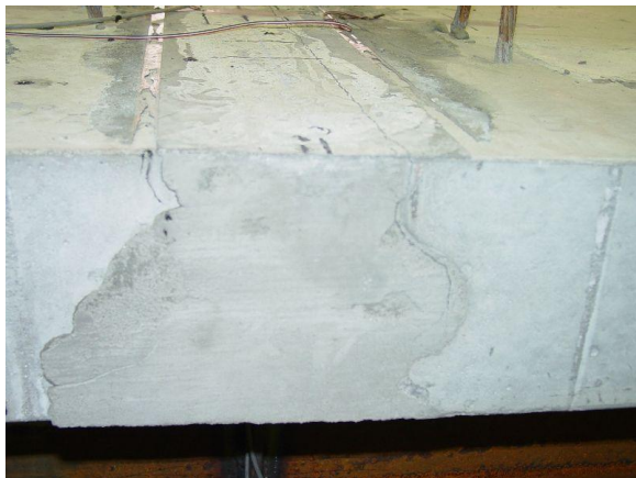
Cracking at closure region
