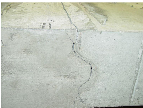
Cracking at closure region
