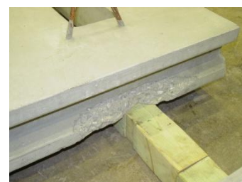
Panel E damaged
