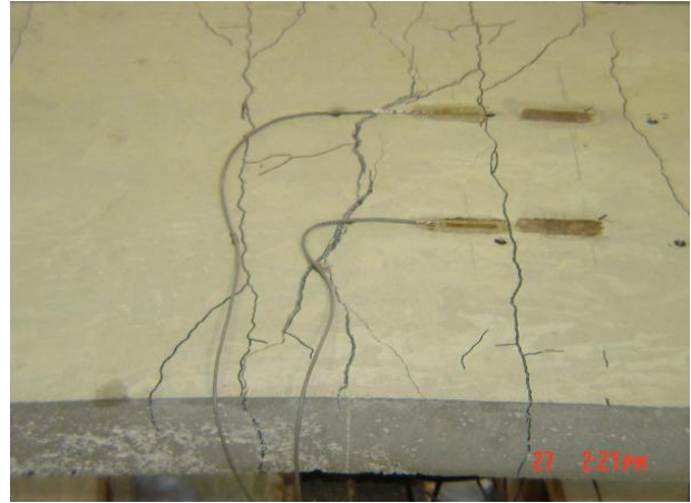
b) Crack pattern over the center support
