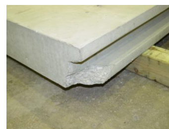
Panel I damaged
